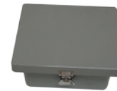
Top of Tank Junction Box
